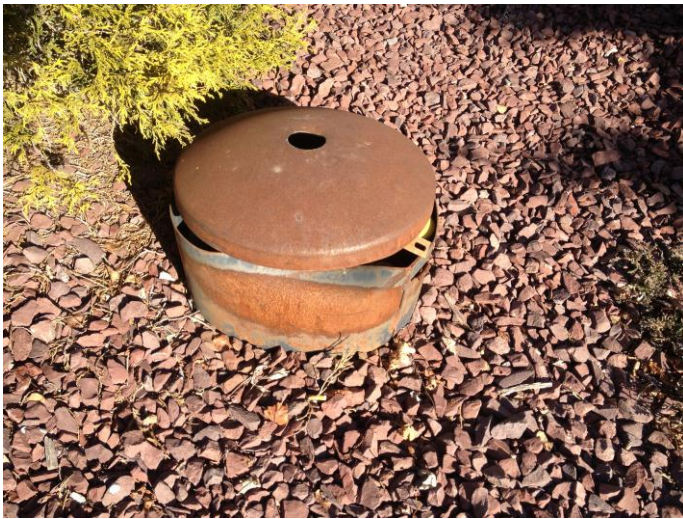
Water meter vault.
