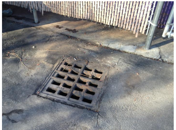
Additional storm drainage catch basin adjacent trash enclosure.
