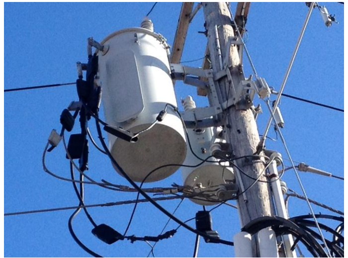
Electric transformers at southeast corner of site.
